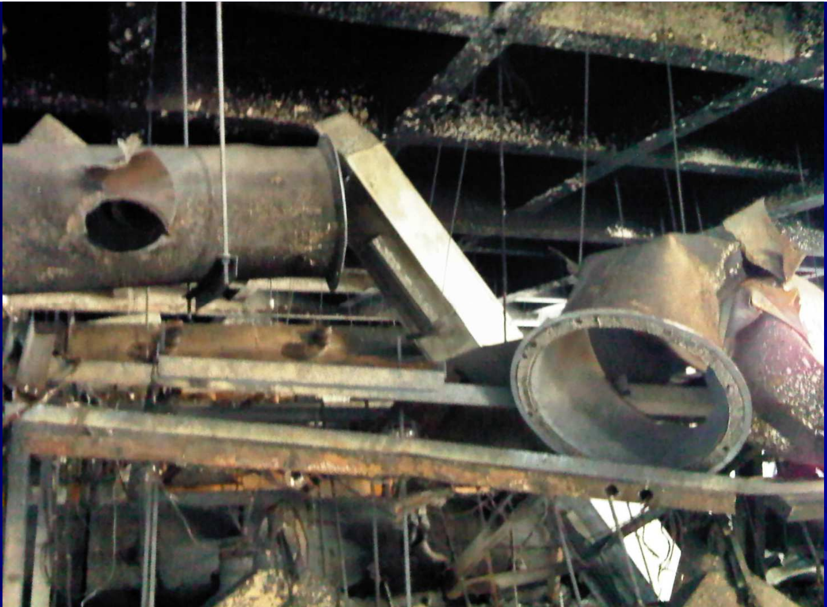
Figure 7-61. Detailed view of damage of dust extraction ducting. From Li et al. (2016)
